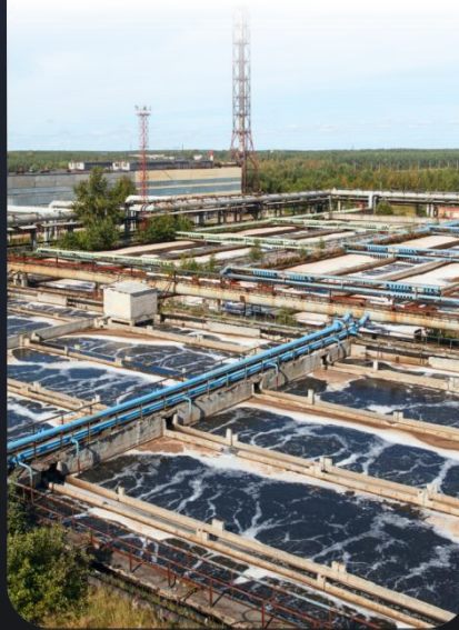
Large water system treatment
